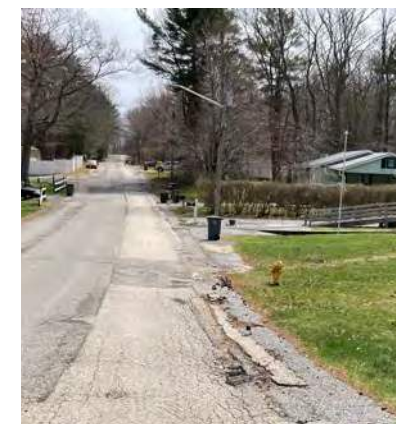
Road conditions on Princeton Street
