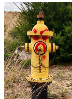
Non-working fire hydrant
