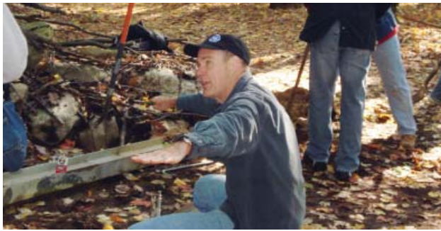
NCLT Director, Jim Walsh led a group of volunteers from DRS Power Technology in a trail work day which included the installation of bollards and chains to prevent unauthorized access to Crocker CA trails by motor vehicles.
